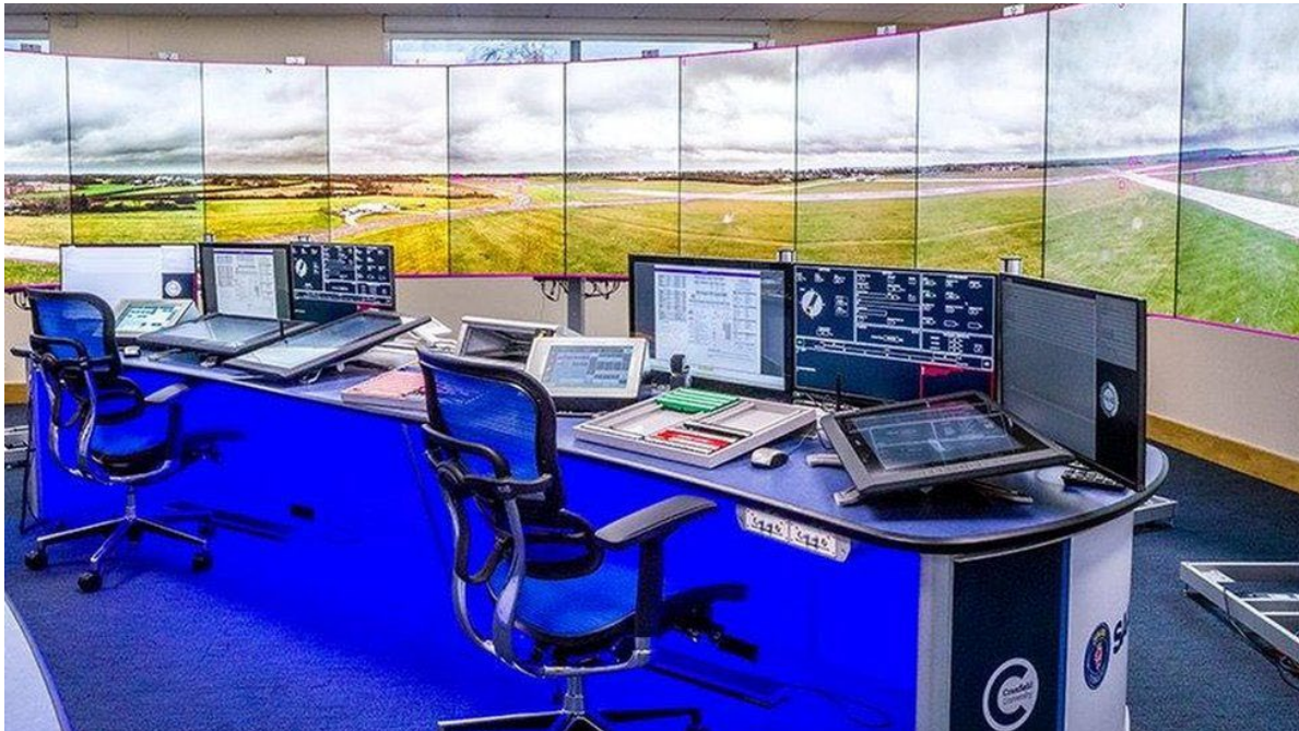
Cranfield University Airport's new Digital Air Traffic Control Centre
